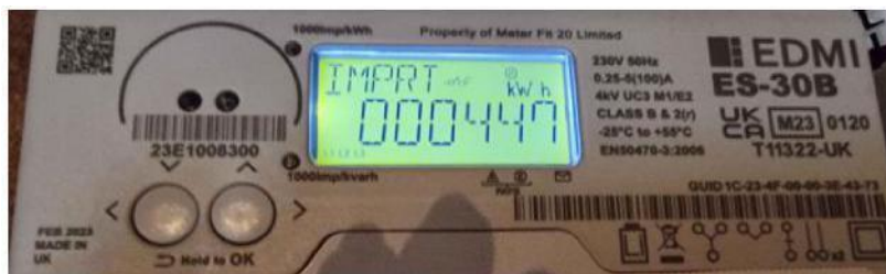
Energy Used 16 th August – 7 th November 2023.
